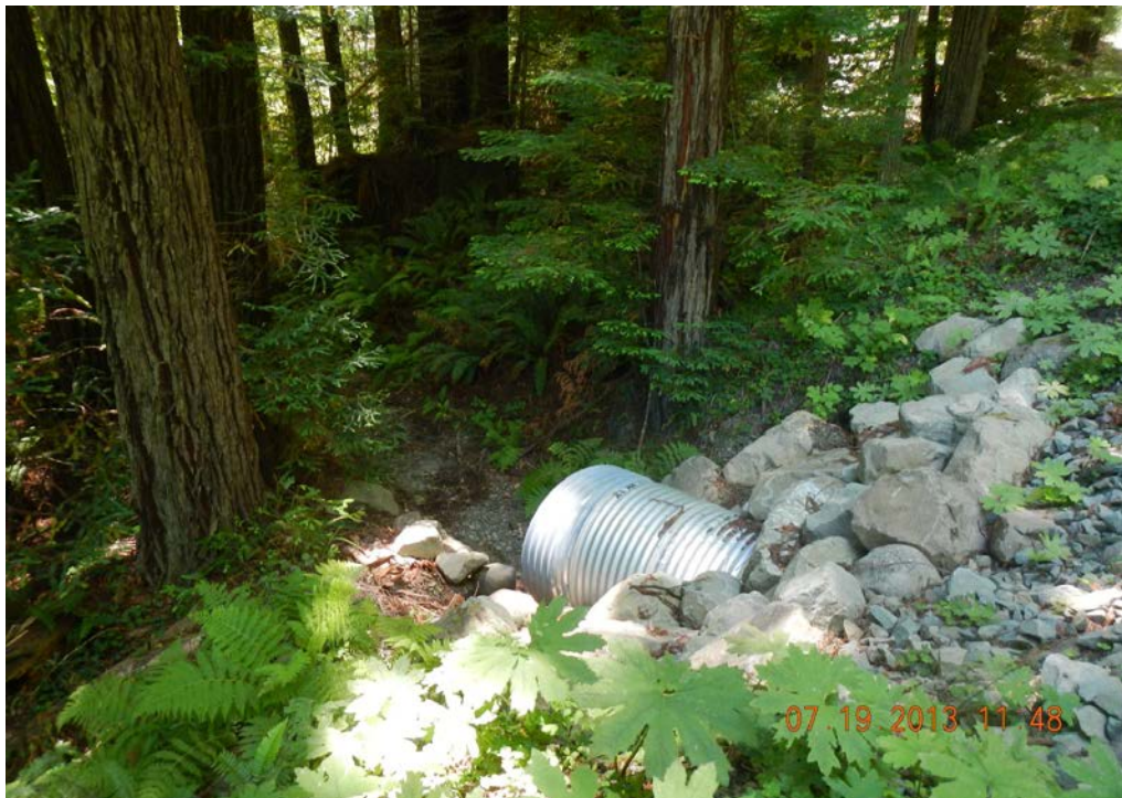
Mitigated exemption, oversize culvert on flat road grade, Yager Creek Basin, summer follow-up inspection
