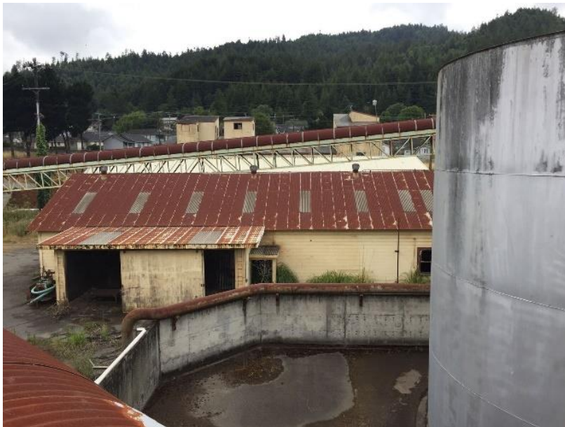
Figure 201 view from the west of the single hipped roof system with corrugated metal roofing and translucent corrugated panels.
