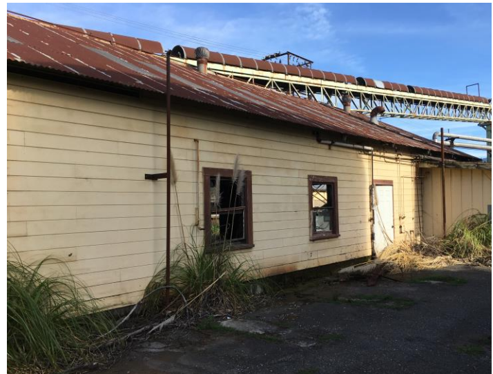
Figure 78 1.D west exterior wall, wood horizontal siding, double-hung windows and frames, standard door to interior. Metal corrugated roofing.
