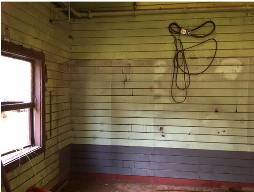
Figure 98 4.A double hung wood window, frame and surround, horizontal interior siding, and floor to roof partition wall.
