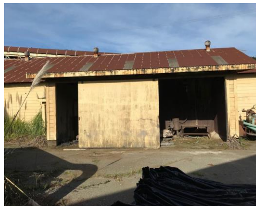
Figure 119 west side facing exterior non-contributing addition with corrugated roofing.
