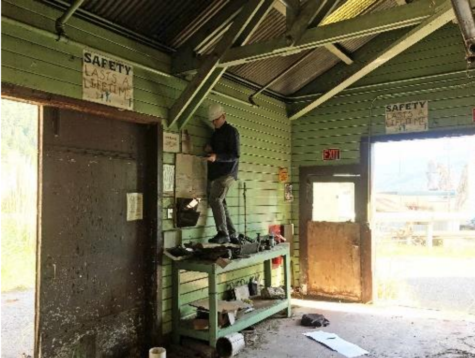
Figure 101 4.D south – east interior corner of building with wood sliding doors, single door, horizontal wood siding, and truss brackets and horizontal chord.
