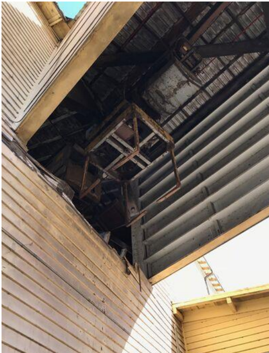
Figure 36 2.G interface of Tunnel #2 with the Manufacturing Building and underside of monorail cab support.
