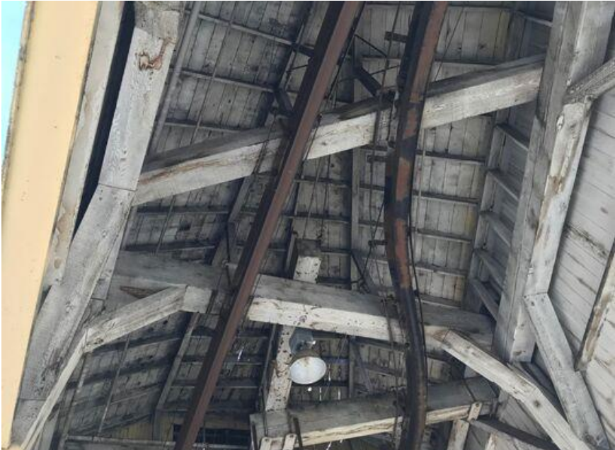
Figure 56 3.H monorail tracks, structural frame of covered area, beams, rafters, electrical light fixture.
