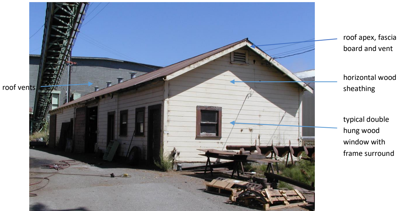
Figure 245 2.A south view of building, side-facing gable, typical double hung wood windows, wood doors, horizontal wood sheathing, vent at apex of north wall.
