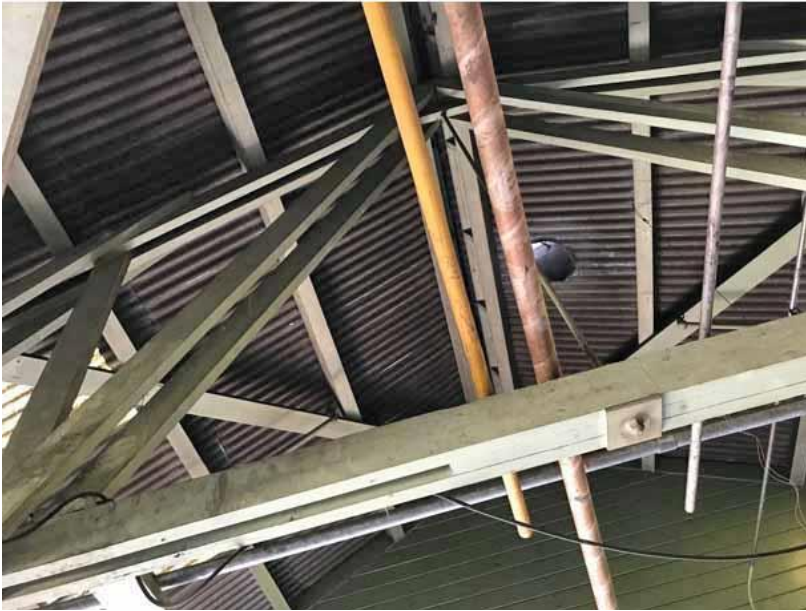
Figure 105 4.H view of truss members, open ceiling, and underside of metal corrugated panels on roof.
