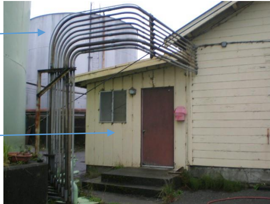
Figure 66 exterior electrical distribution panel.
