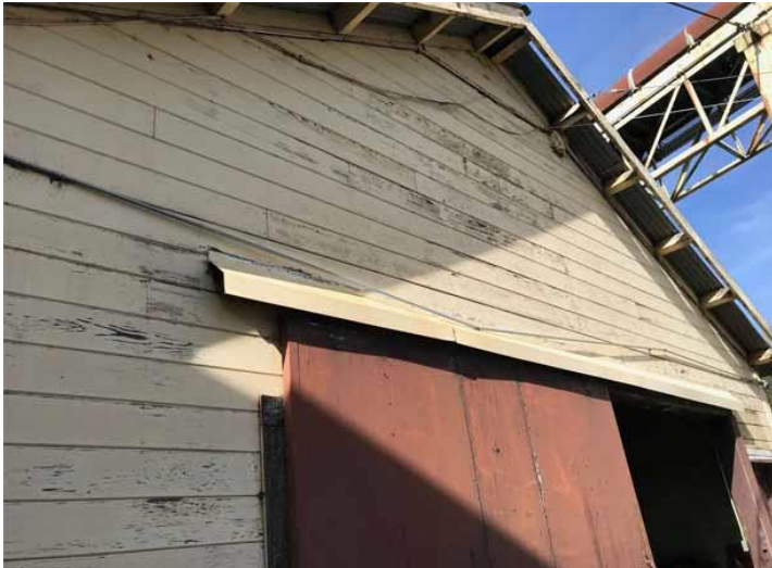
Figure 82 north facing side gable double sliding wood door with tracks cover, horizontal wood sheathing, open eaves.
