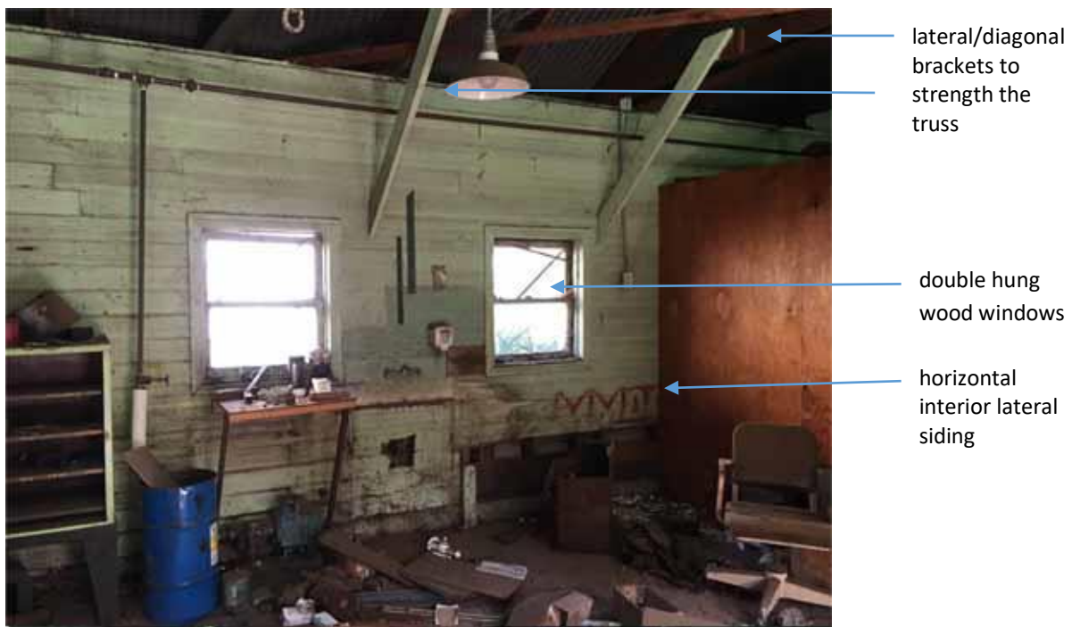
Figure 262 4.A interior double hung wood windows with frame and surround, two lateral/diagonal brace.
