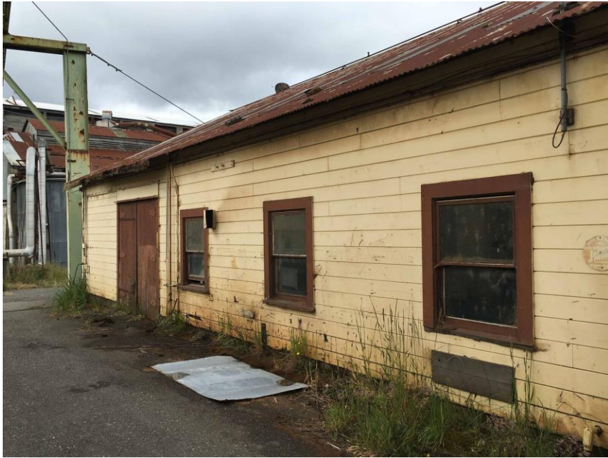
Figure 86 2.B east facing exterior wall from southeast, sliding wood door, double hung windows, horizontal wood sidings, metal corrugated roofing.
