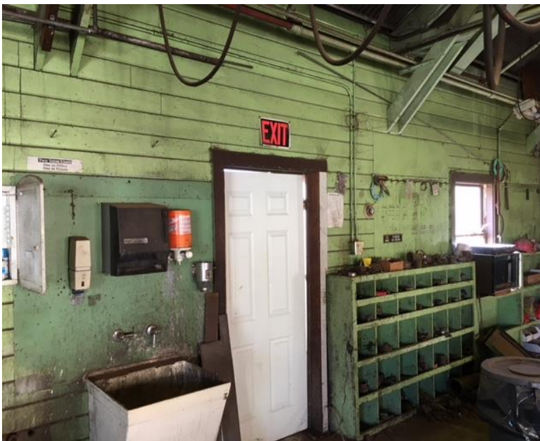
Figure 93 3.C typical wood door with frame and surround, sink, and wood cabinets and shelves.
