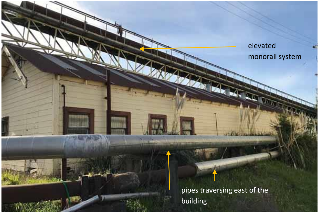
Figure 253 2.C monorail system running above to the west of the building, pipes along the east side of the building.
