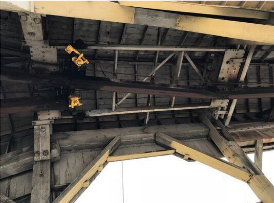
Figure 55 3.G monorail tracks and column bracket supports.
