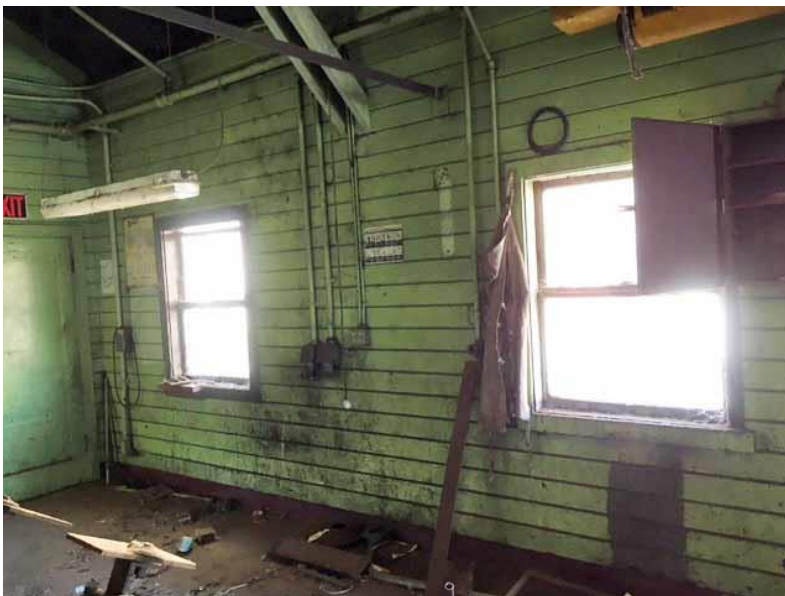
Figure 102 4.E double hung wood windows, frame and surround, horizontal wood siding, at the west wall.
