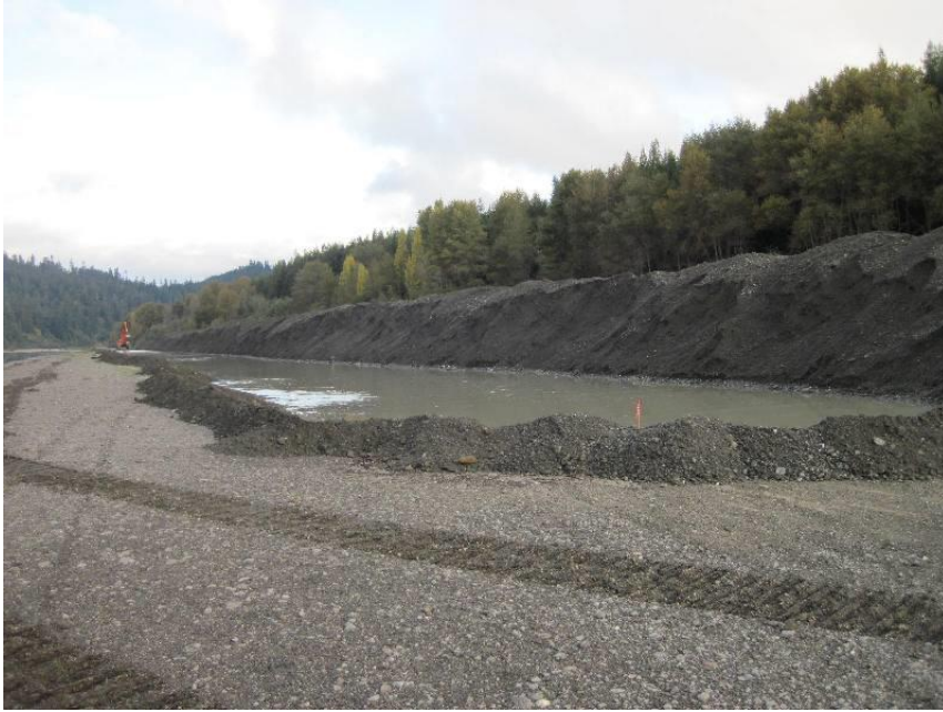
Figure 6. Excavator and trench on Truck Shop Bar during 2012 operations (for example of operations).
