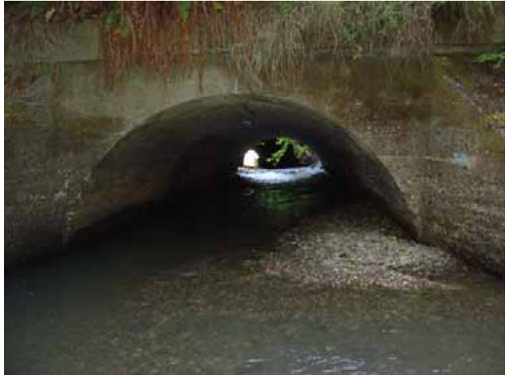
Photograph 5-11. Lower Poison Oak Creek highway crossing as an example of early construction practices at stream crossings—this culvert is not a barrier to passage during low flows
